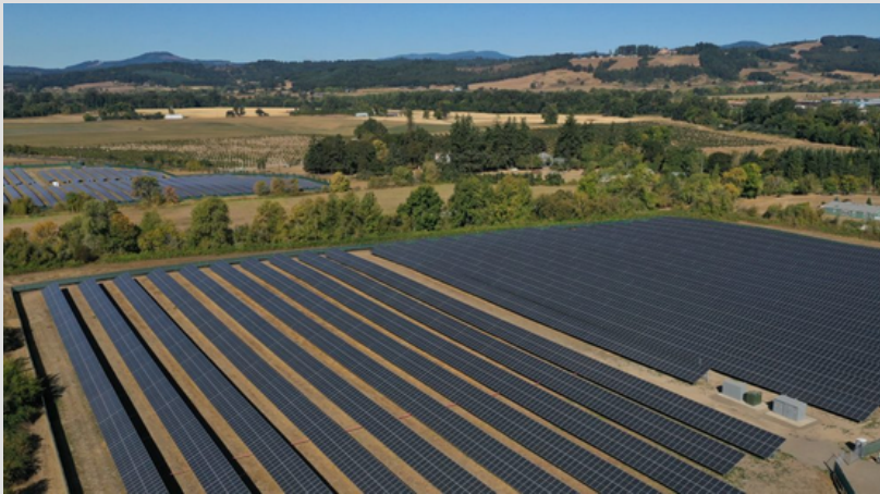
Red Prairie Community Solar Project
